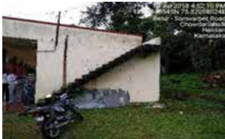
MR Aided High school, Sakaleshpura-Staircase without railings
