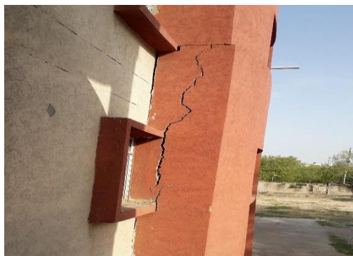
Cracks in walls of Research Hospital building
