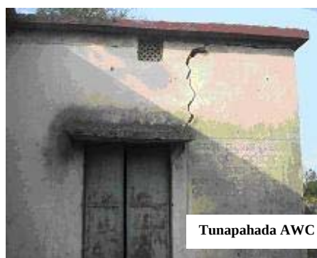
Photograph showing unsafe Anaganwadi Centre at Tunapahad
