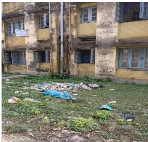
Pic 2.1.22: BMW disposed openly in DH compound
