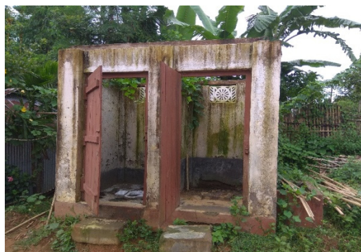
Photograph 2.2.6: Broken toilet in Haripur 12 Card-under Dumburnagar ICDS Project
