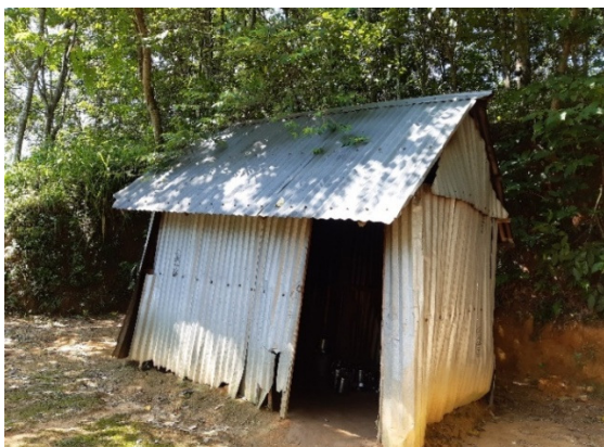
Photograph 2.2.3: Broken kitchen in Lungapar AWC under Dukli ICDS Project
