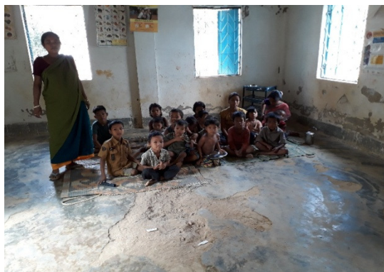
Photograph 2.2.1: Broken floor in Taraban colony AWC under Dumburnagar ICDS Project
