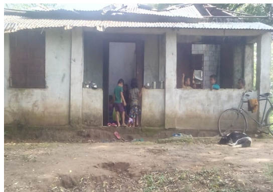
Photograph 2.2.2: Broken Roof in Das garia AWC under Hezamara ICDS project
