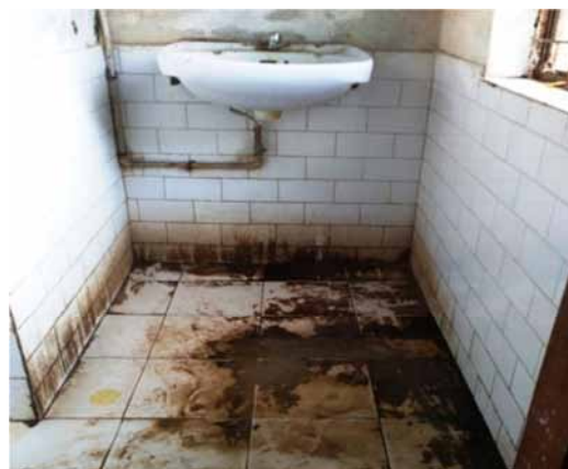
Poor cleanliness -SDH, Gandacherra
