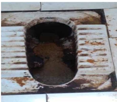
Poor cleanliness-SDH, Gandacherra
