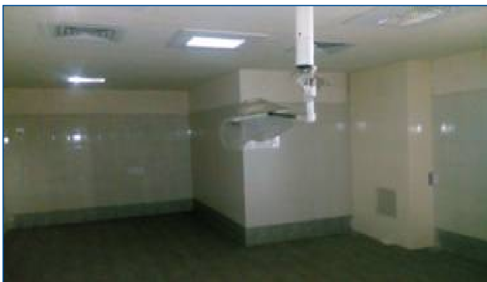
Picture 14: Non-operational OT at CH Surat (25.07.2015)
